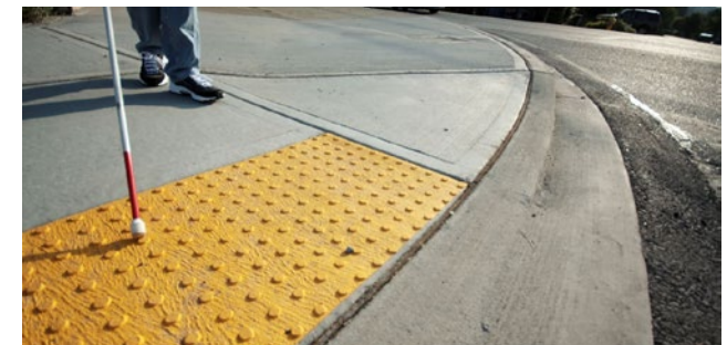
Figure 68: Example of tactile paving to facilitate movement for people with visual impairment
